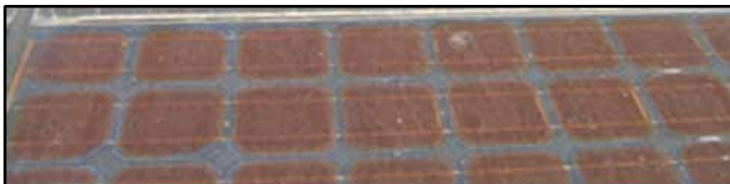
Figure 21: Encapsulant browning due to UV in a hot-dry condition (Site: Phoenix, Arizona; Arco Solar M55 modules installed in 1985 and still operating after 26 + years).
