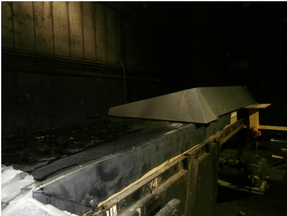
Figure 6 – Figure Illustrating Damage to Roof Surface.
