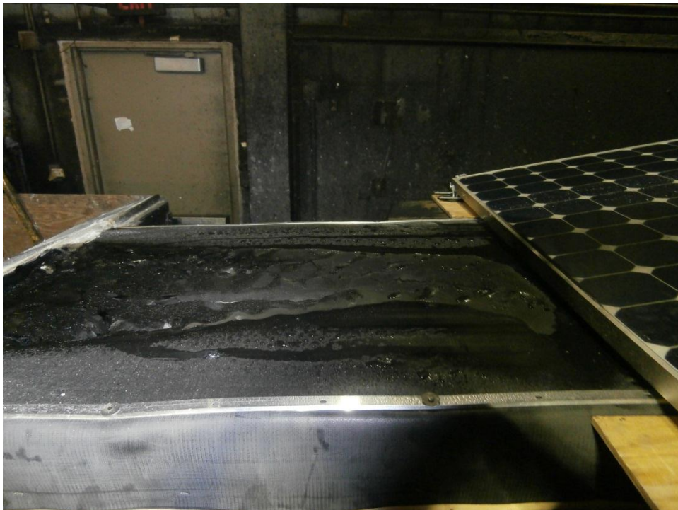
Figure 8 – Figure Illustrating Damage to Roof Surface.
