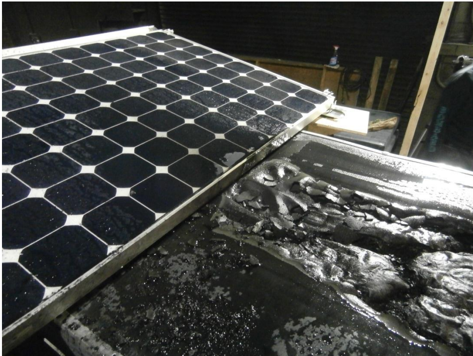
Figure 3 – Figure Illustrating Damage to the PV Module and the Roof Surface.
