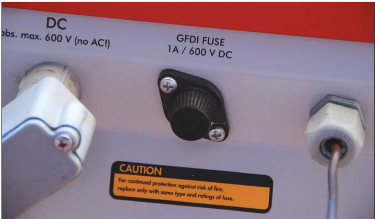
Photo 4. Ground-fault fuse on high-voltage inverter
