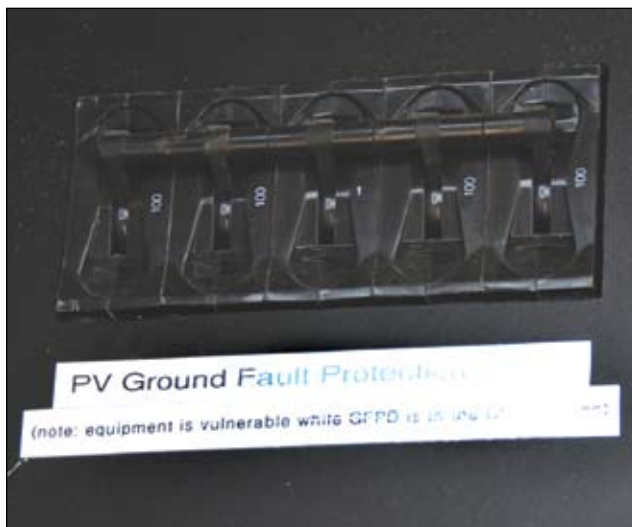
Photo 3. Four-pole, ground-fault protective device for 48-volt PV system
