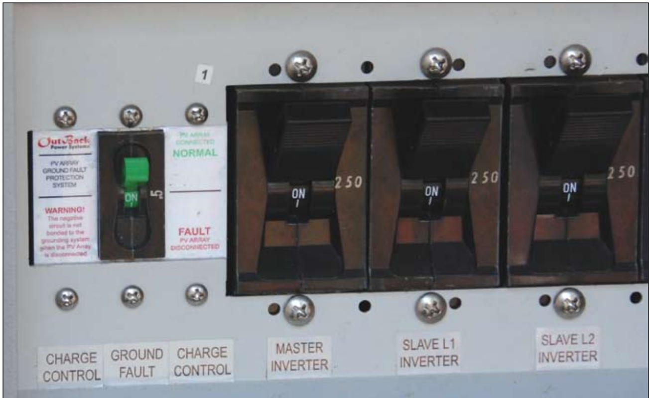
Photo 2. Two-pole, ground-fault protective device for 48-volt PV system
