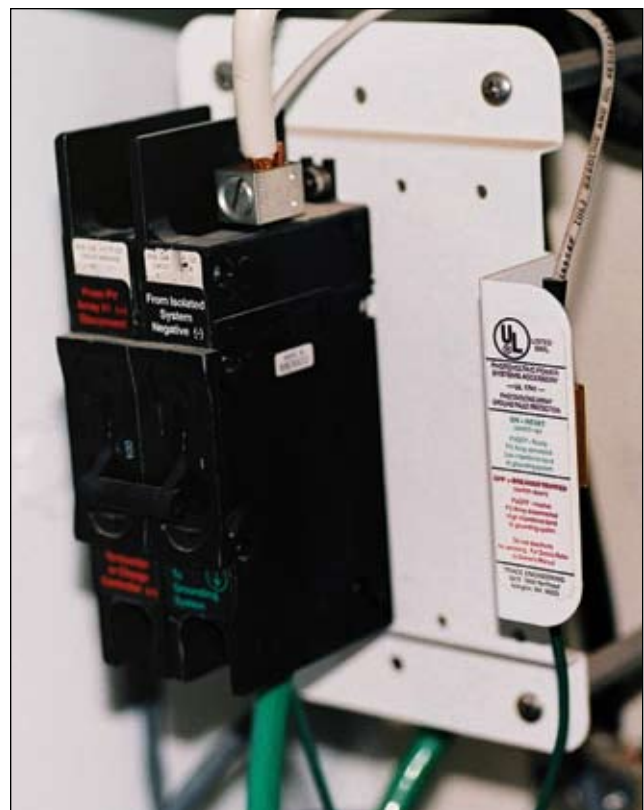
Photo 1. One-pole, ground-fault protective device for 48-volt PV system
